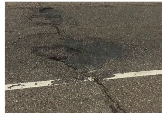
Poor pavement along a state highway
